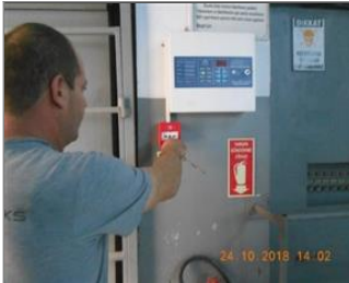
External photo(s) of the production unit(s) fire alarm testing.JPG
